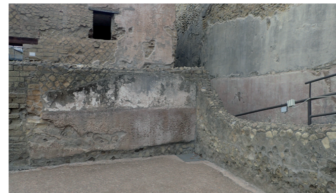
Fig. 3B. A wall in the garden of the House of the Deer showing the distinct change in decoration from the cocciopesto lining at the bottom.
